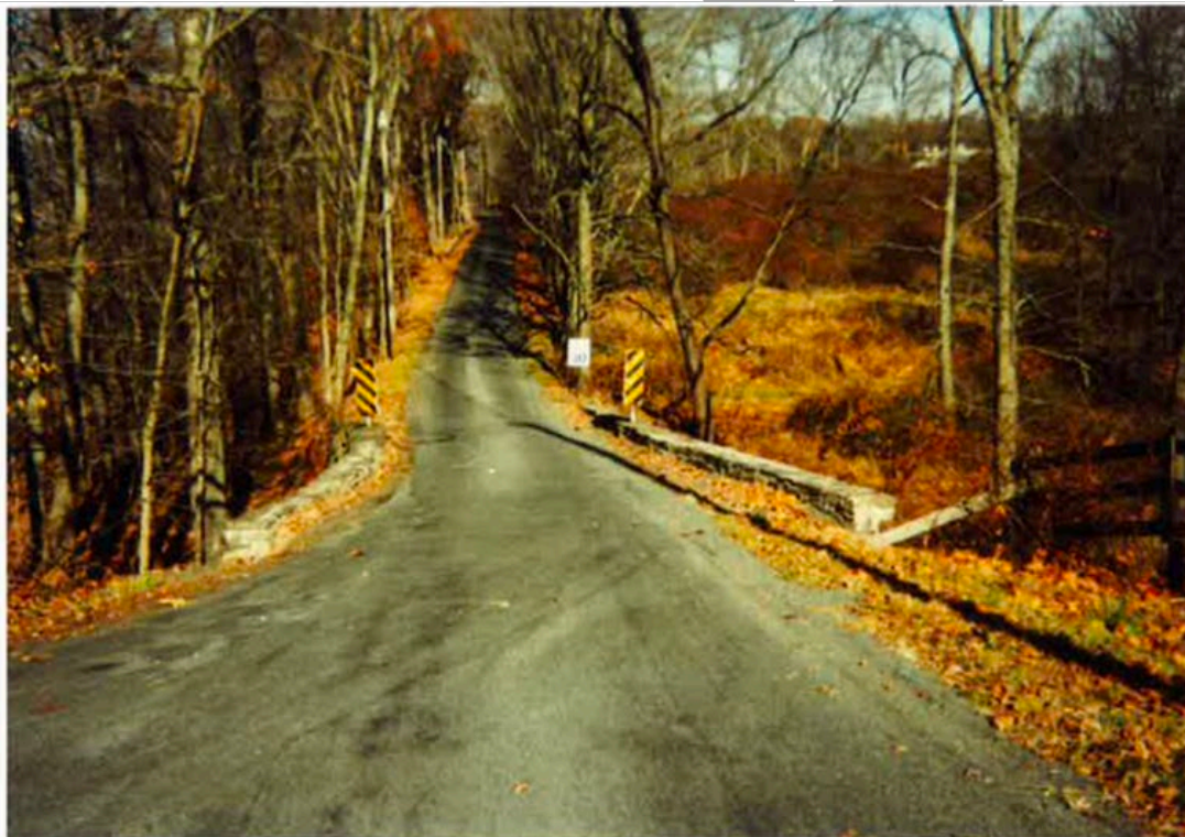
Illustration 14: Top view November 1992 taken before the parapets were raised. Lower view November 1998 taken after the parapets were raised. Pine Hill Road, view facing north from Rosemont Ringoes Road (Route 604). 12
