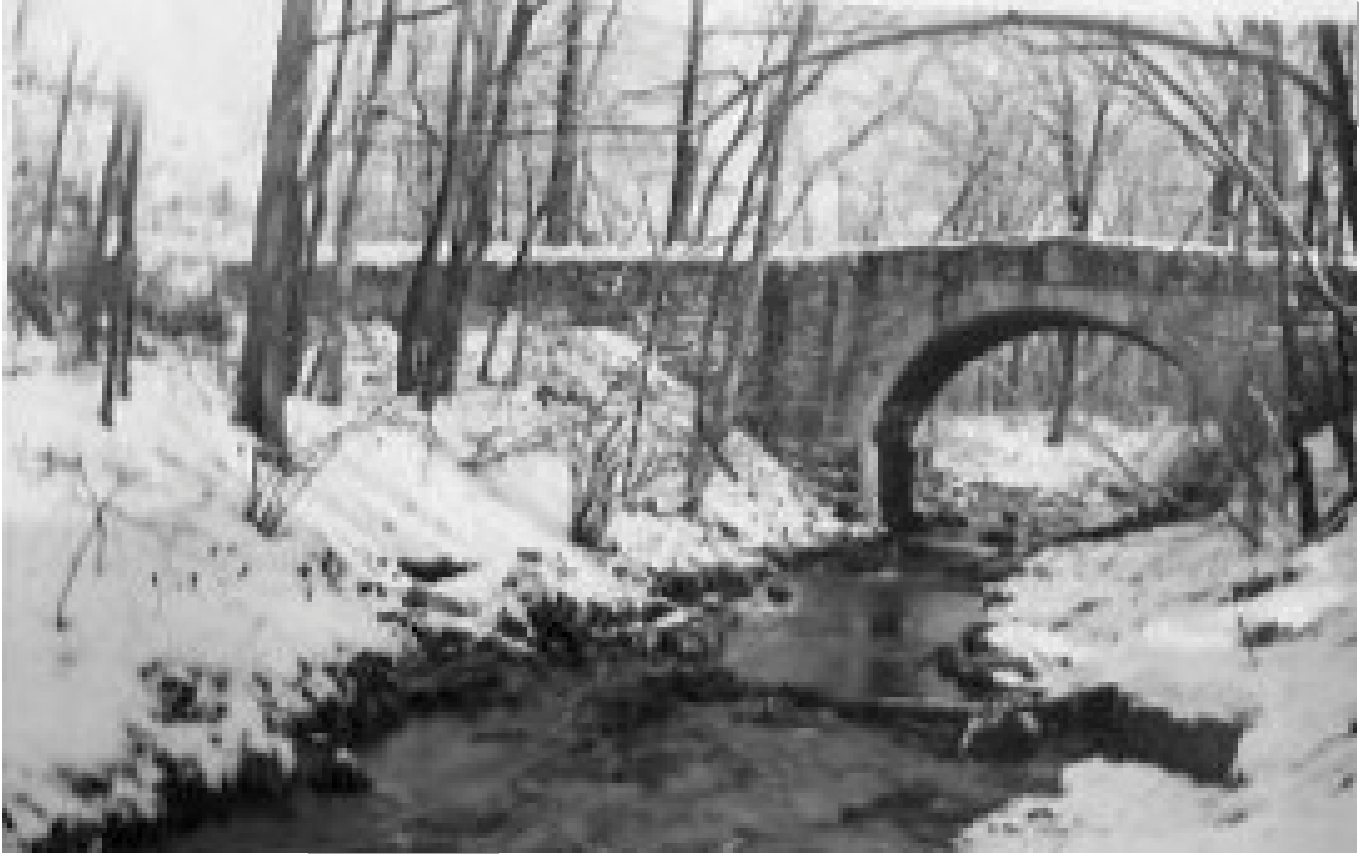
Illustration 7: Early 1940's photograph of the downstream side of the Pine Hill Road Bridge by Georgia Cotton who lived in the miller's house near Pine Hill Road. Complements of Gary Hinesley
