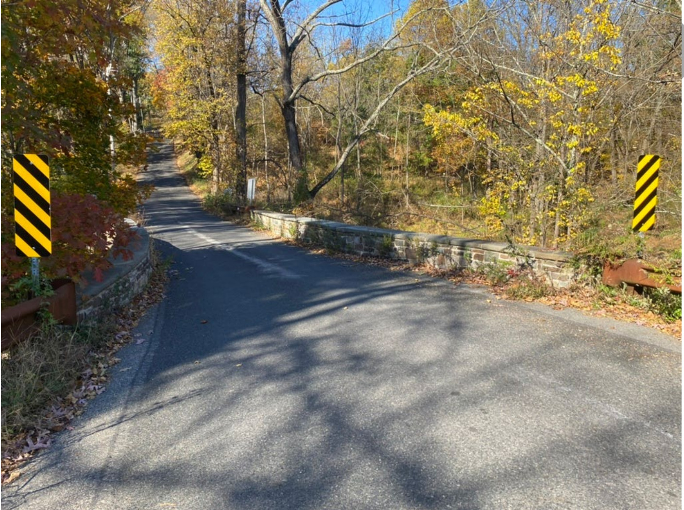
Photo 2: Pine Hill Road and the stone arch bridge, View facing north, showing the reconstructed parapets.
