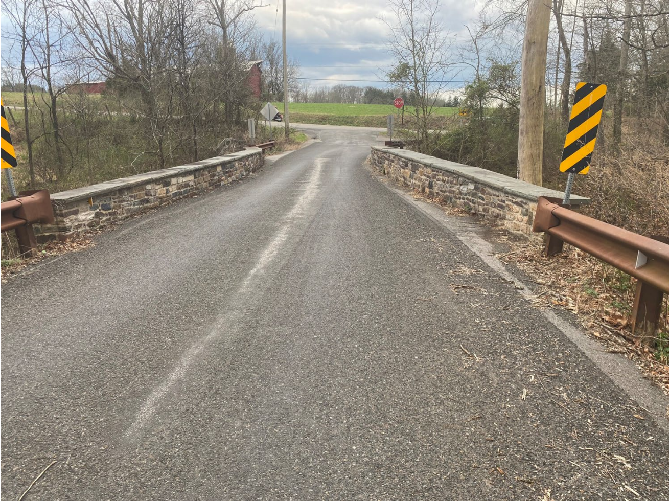
Photo 1: Pine Hill Road and the stone arch bridge, View facing south, showing the reconstructed parapets.
