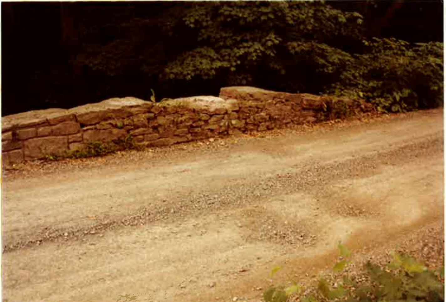
Illustration 10: 1980. West parapet with missing capstone. 8
