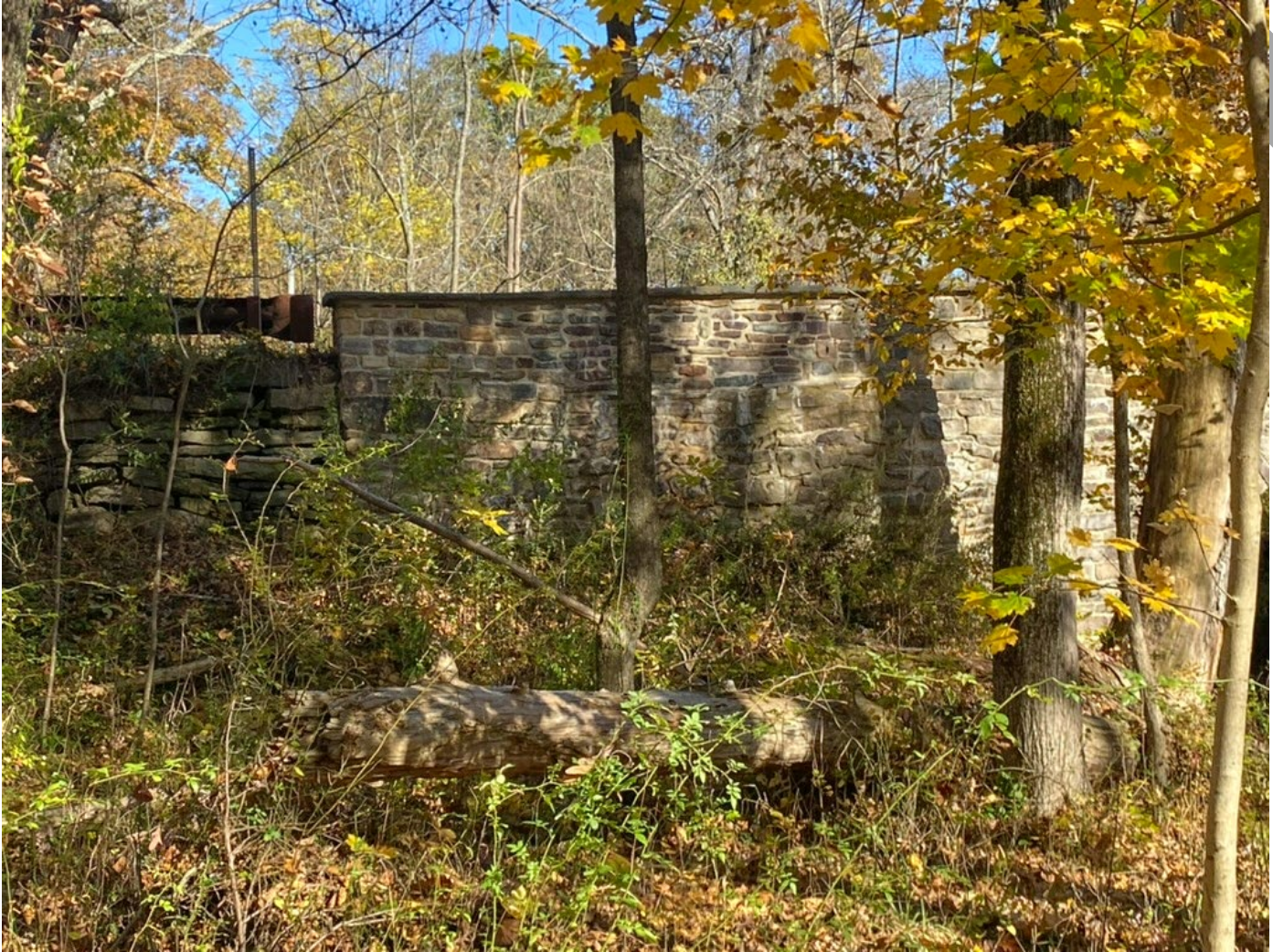
Photo 8: West (downstream) side of the Cold Water Bridge, View facing east, showing the northwest wingwall with raised parapet and a section of wall with no pointing.
