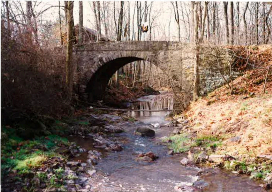
Illustration 13: November 1992. West downstream side of the bridge (upper view) and east upstream side of the bridge (lower view). 11
