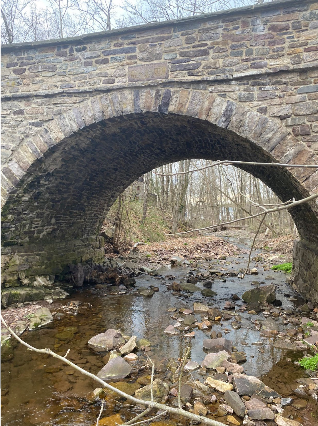
Photo 4: East (upstream) side of the Cold Water Bridge. View facing west, showing the raised stone bases.
